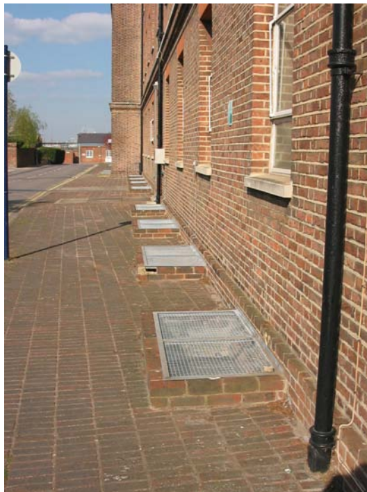
Figure 7.4: Ground level vents, 'B' Block
