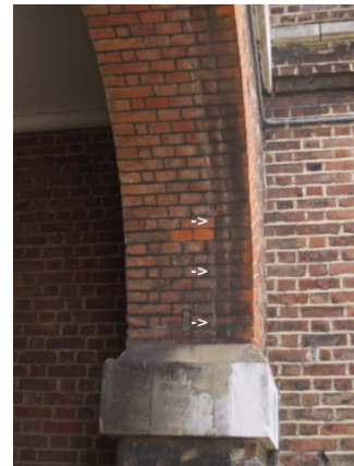
(b) Brickwork 'scarring'
